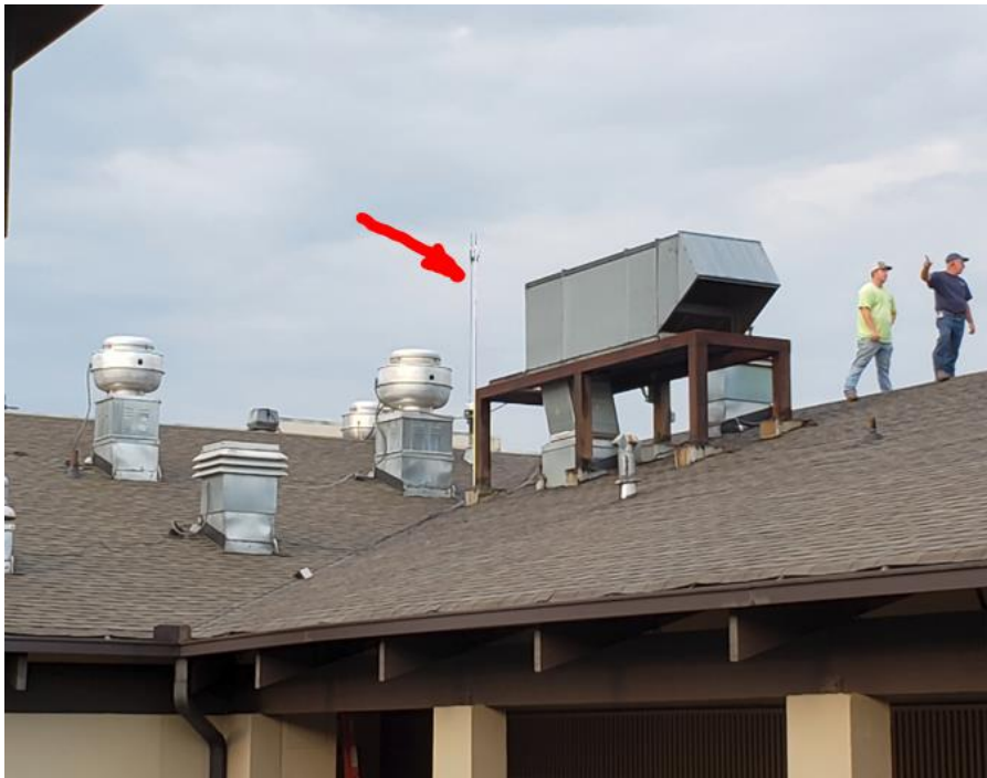
Electrical Conduit Mount attached to AC unit.
